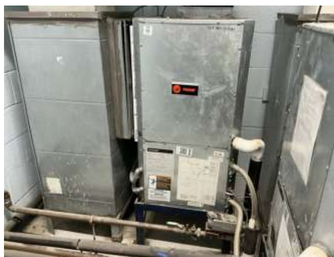
24 - WATER SOURCE HEAT PUMP
