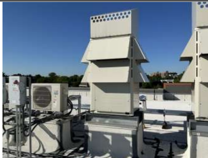
26 - VRF SYSTEM INVERTER
