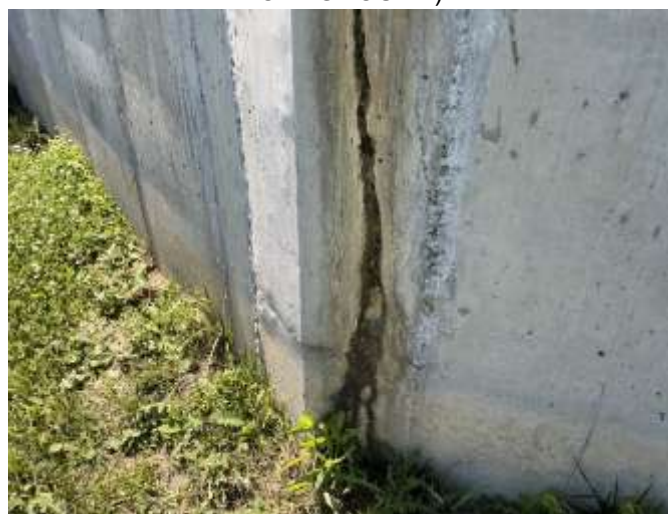
36 - RETAINING WALL (CRACKED)
